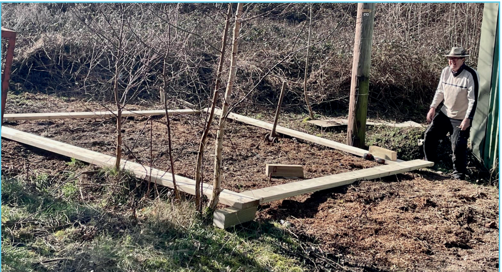
Our wonderful engineers building a shrub nursery for growing native species to plant around the reserve.
